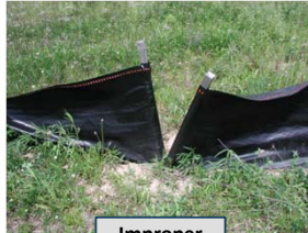
Improper Joint Gap
