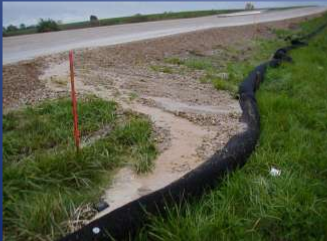
Channelized flow coming off the saturated roadbed
